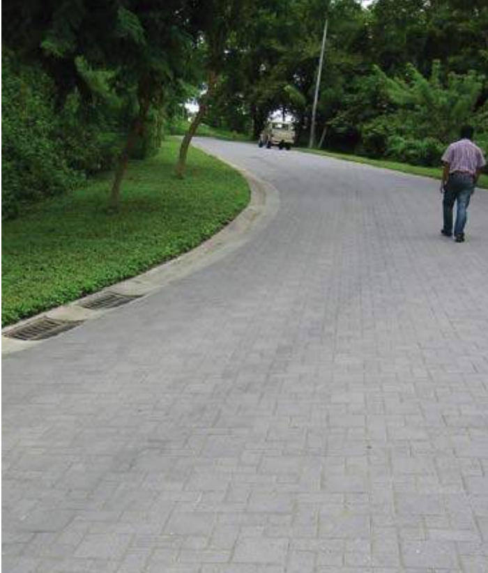
Figure 2. This Costa Rican road reaches up a mountain at maximum 25% slope. The paving pattern imitates a herringbone which is recommended for sloped applications. This photo shows a four year-old pavement.
